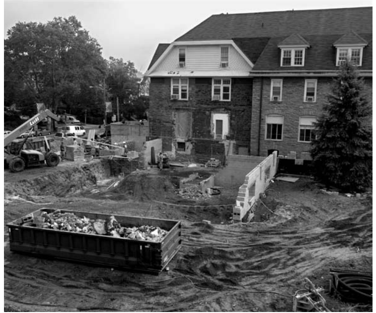
The administration building is gone! This shot overlooks construction from the west and toward HMS's main building, with 44th St. and Baltimore Ave. at the upper left.
